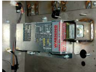
POWER SWITCH ON AC SUPPLY
