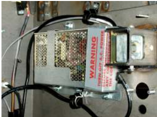
POWER SWITCH ON DC SUPPLY
